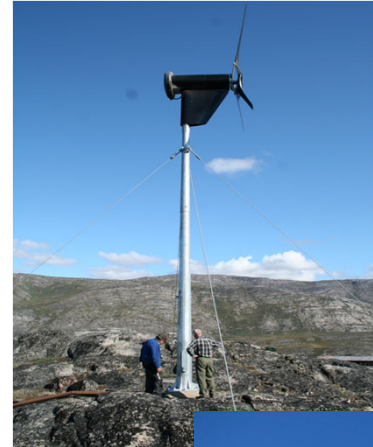
6 kW Proven wind turbine Proven WT 6000 (Kingspan)
